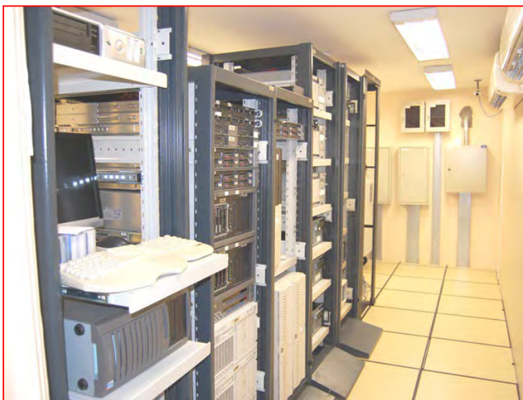
Fig. 7.4: Sala Principal do Data Center
