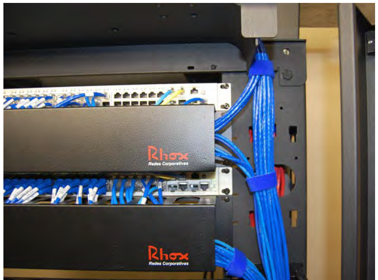
Fig. 7.18: Switches OS-LS-6248 no rack do DS
